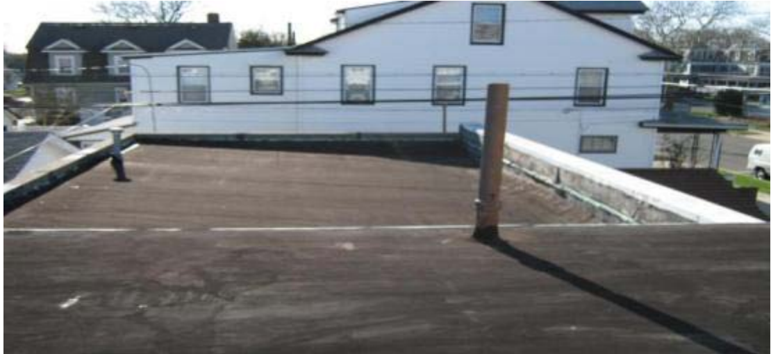
Roof photo indicating wear and exposed fiberglass.
